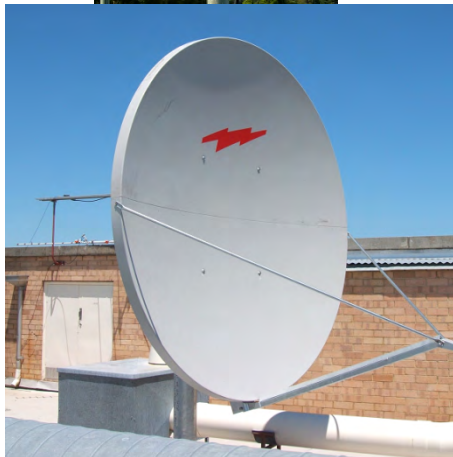
2.4 m antenna TWSTT
